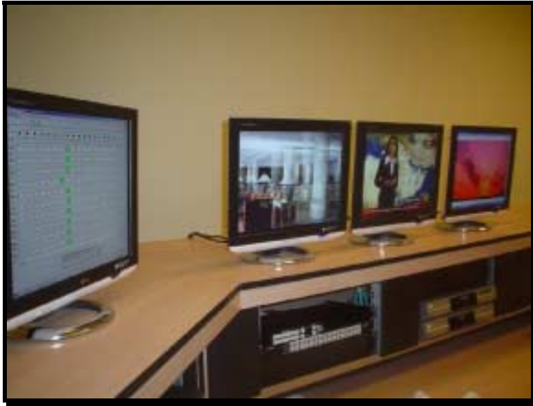
Control Room with Matrix Switchers
